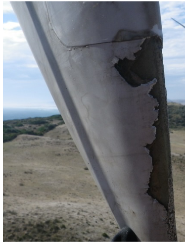
Figure 1. Typical damage caused by erosion on a rotor blade.
